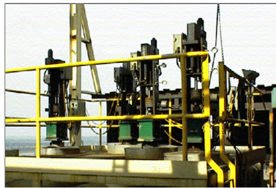
Figure 2: KCP&L Superheater Bypass Valves
