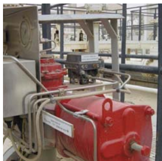
Qatar Petroleum mounted a Fisher FIELDVUE Digital Valve Controller on a Tyco emergency-shutdown (ESD) valve at its gas processing station in Dukhan.
