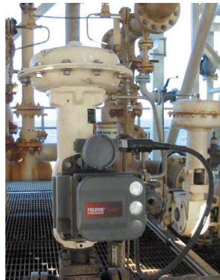
FIELDVUE DVC6000 instruments with advanced diagnostics monitor the performance of 52 control valves on the Griffen Venture FPSO. The facility draws, stores, and off-loads oil and gas from sub-sea wells.
