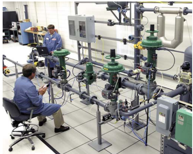
Fisher engineers designed the new PlantWeb™ Performance Laboratories used in Marshalltown (USA), Singapore, and Cernay (France).
